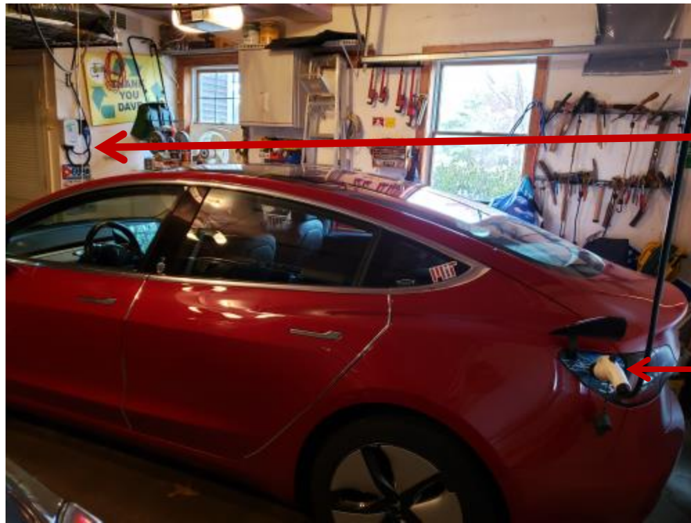
Roper garage 7.2-kW charging station
